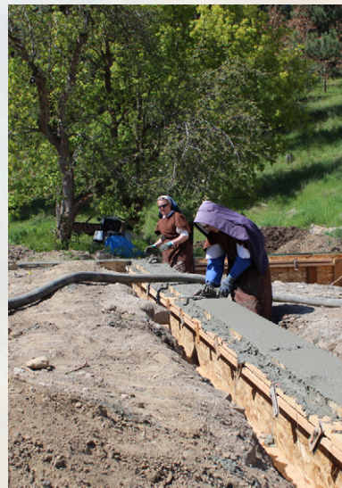
New life skills for novices and postulants: spreading concrete for the footings at the novitiate project site.
