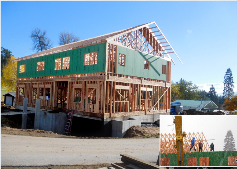
City of Mary convent construction. Inset: The men putting up the trusses in snow and cold rain! They had to do it that day because the crane was rented for that day at several hundred dollars an hour. (!!)
